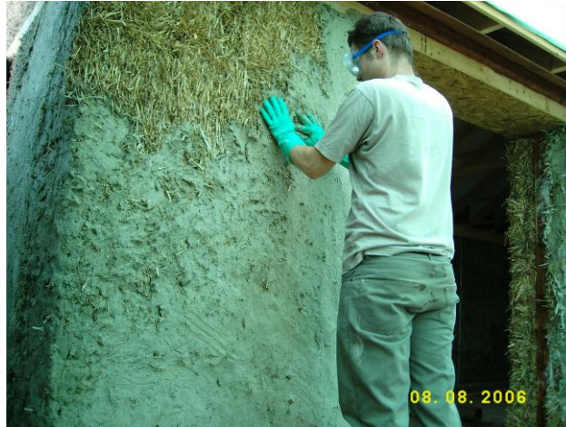
Applying the first coat of lime render by hand at The Straw Bale Cabin
