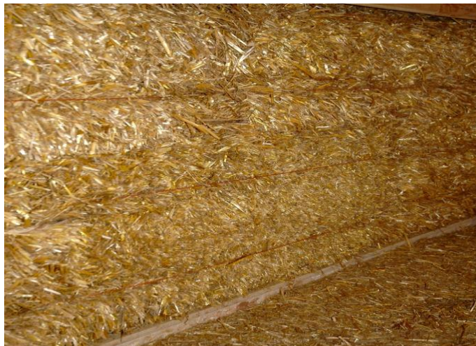
Photo courtesy of Jim Carfrae – straw bales stacked on edge at his straw bale home, Totnes, Devon – the strings are visible inside and out
