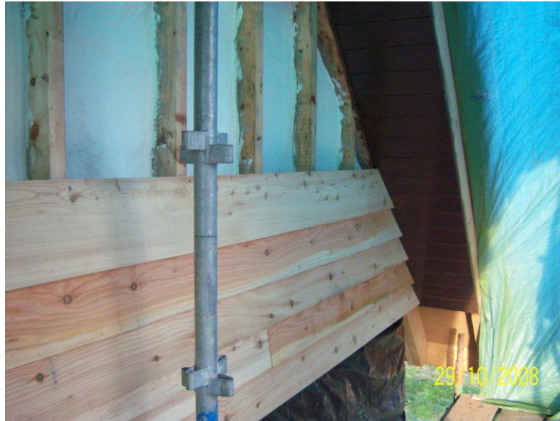
Larch boards forming a ventilated rain screen over clay plastered straw bales at The Straw Bale Cottage
